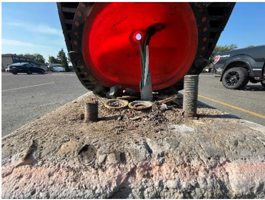
Photo 3: Sheared anchor rod
