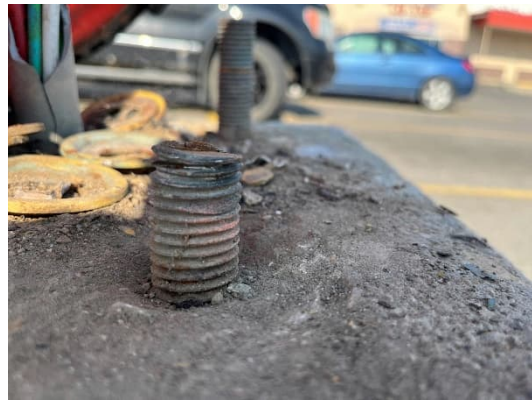
Photo 4: Bent anchor rod
